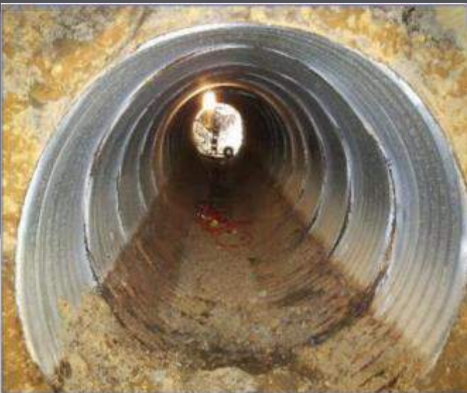
Damage to the seams and corrosion present.
